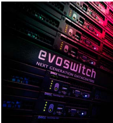
LeaseWeb’s rapidly expanding Data Centre
